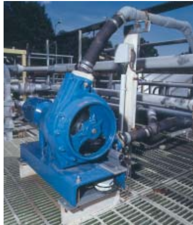
Z pump in neutralization of effluents
