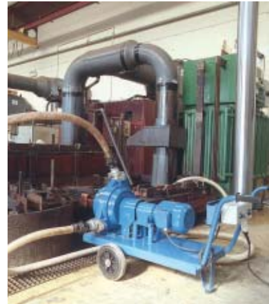
Z pump in draining of wells
