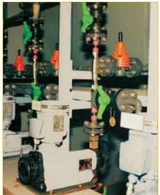
Ferric chloride pumping in purification station
