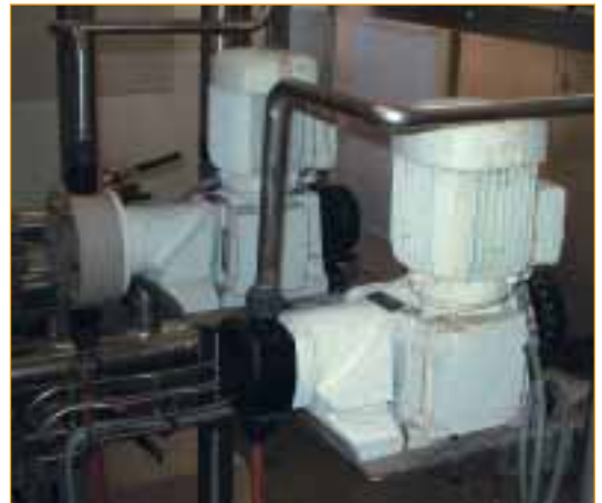
Metering of soda and acid
